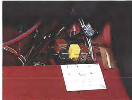
Fuses under rear seat
